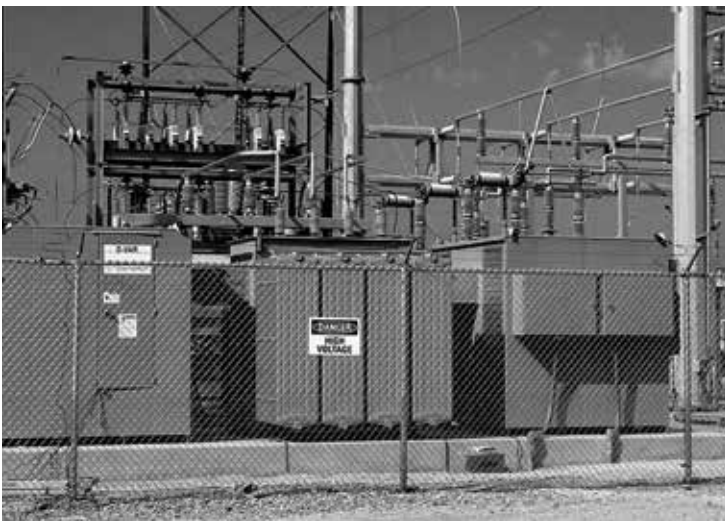
Example of a 8 MVAR D-VAR system, which is 30 feet long by 11 feet wide
