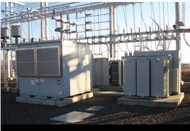
Dynamic D-VAR solution regulates and stabilizes voltage levels by injecting VARs into the power grid at precise locations where voltage problems can occur. The D-VAR pictured is not identical to the Entergy deployment at Natchez. (Photo courtesy of American Superconductor)
