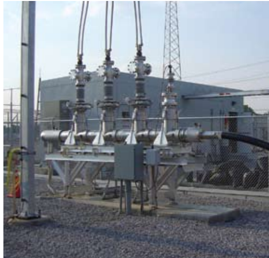
Southwire Triax HTS cable termination installed at American Electric Power's Bixby Substation. Photo courtesy of Southwire Co.
