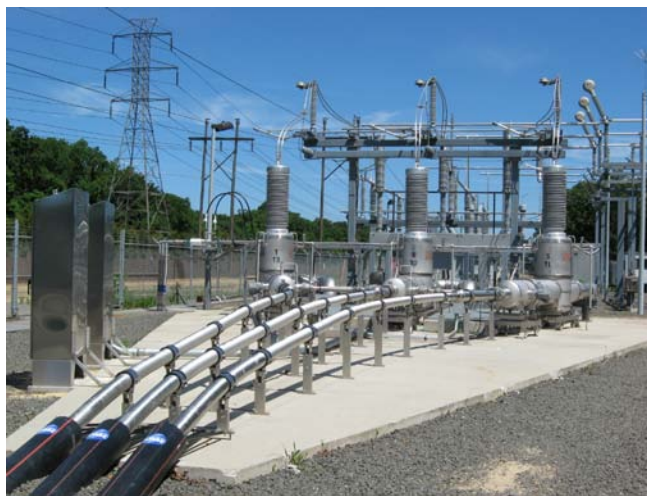
Figure 1: 138 kV AC superconductor power transmission cable operating since April 2008 in Long Island Power Authority's grid (photo courtesy Nexans)
