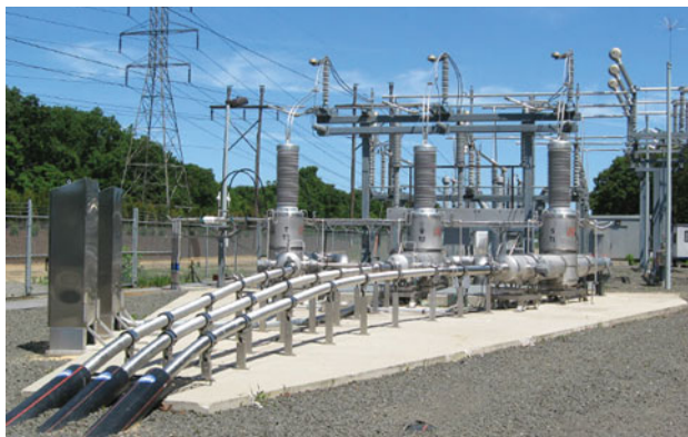
The Long Island Power Authority has been operating, since 2008, a cable system manufactured by Nexans that utilizes AMSC's high-temperature superconductor wire and an Air Liquide cooling system. Energized in April 2008, this is the world's first superconductor transmission voltage cable system, which is capable of transmitting up to 574 MW of electricity and powering 300,000 homes. Photo courtesy of AMSC.
