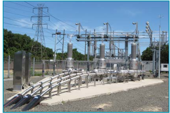
Superconductor Transmission Cable System on Long Island.
