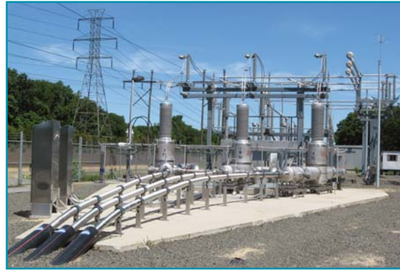
Superconductor Transmission Cable System on Long Island.
