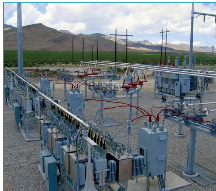
AMSC Transmission SVC Deployment in Western United States.
