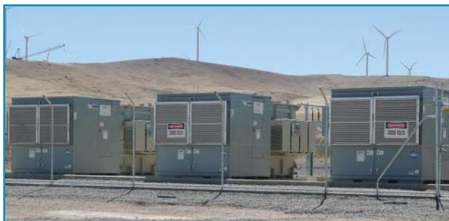
D-VAR® System Installation at Hallett Wind Farm in Australia.
