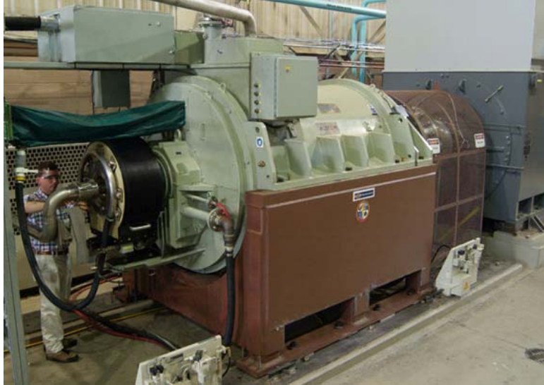
Figure 1: 5 MW HTS motor coupled to two GE 2.5 MW load motors at CAPS
