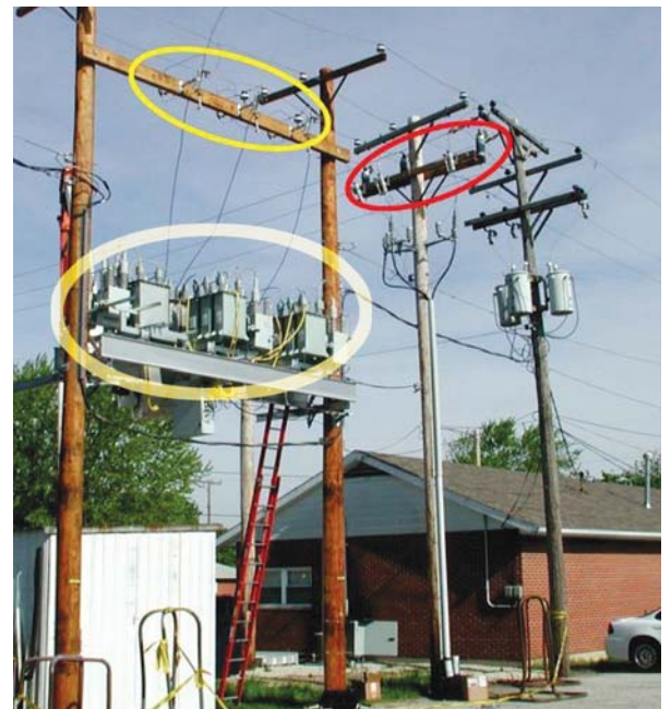
Connection Details: The PQ-SVC system highlighted above was connected to the 13.2 KV distribution primary circuits immediately outside customer's service entrance, using a standard voltage regulator platform. The utility installed one current sensor on each phase pointing at the load (circled in red). Utility disconnect and line to ground fault protection was provided by 3 cutouts using 100A "T-type" fuses (circled in yellow).
