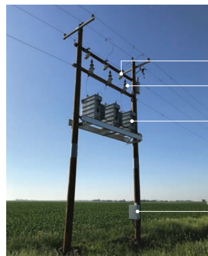
Fuse Vacuum Switch AMSC Power Electronic Units AMSC Control Unit
